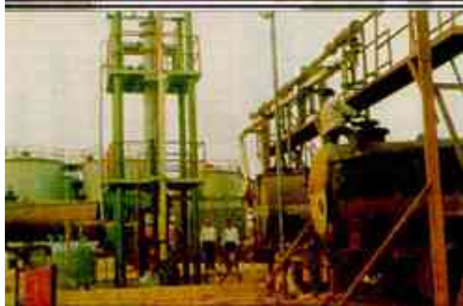
Sludge Dewatering System of a Distillery Unit (above) Hydrochloric Acid Absorption / Handling system of a Caustic soda Industry (below)
